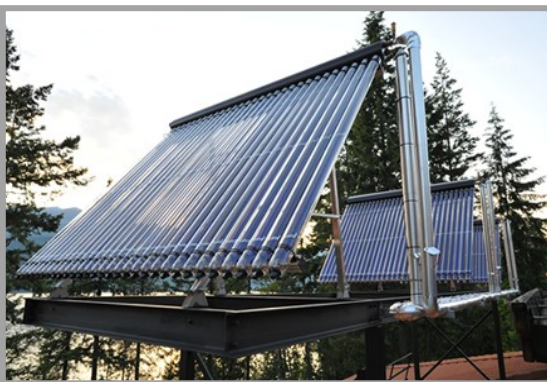
Solar Thermal panels at Yasodhara Ashram
